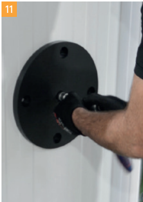
11 Securely fix reinforcement arm backing plate on other side of the wall.
